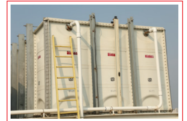
84,000 litre of tank installed in Leela Business Park, Mumbai
